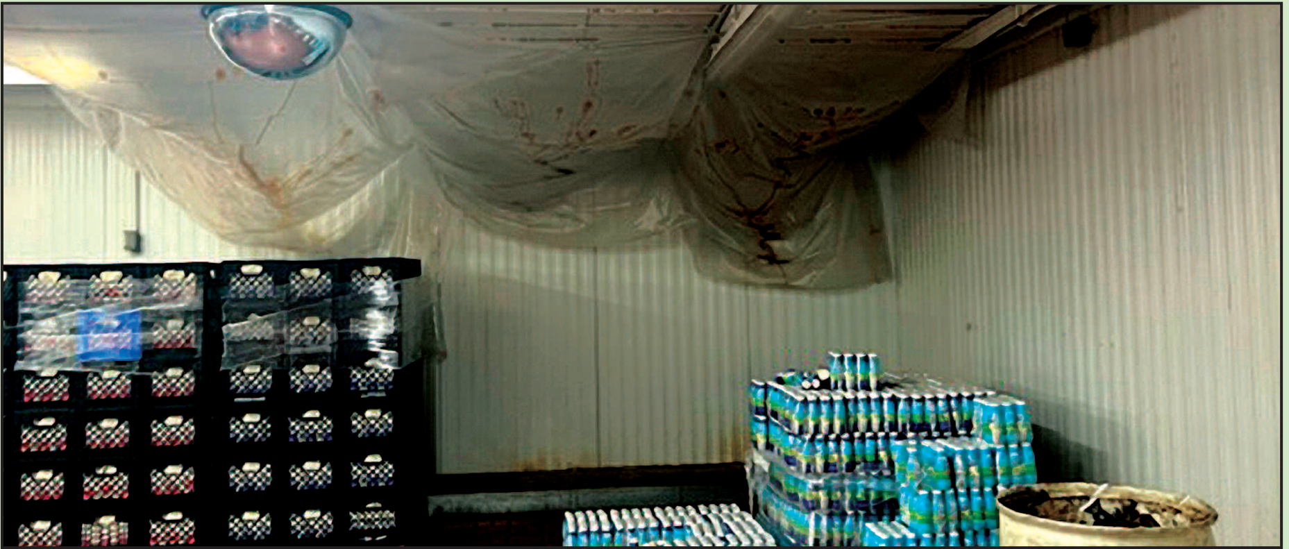
To block rain water from a leaky roof from dripping on cases of milk, heavy clear plastic was haphazardly attached to the ceiling and walls at this cold-storage locker in Franklin Park, Illinois operated by Borden-Select. Black mold has thrived on that plastic. Enough to gag a maggot!
