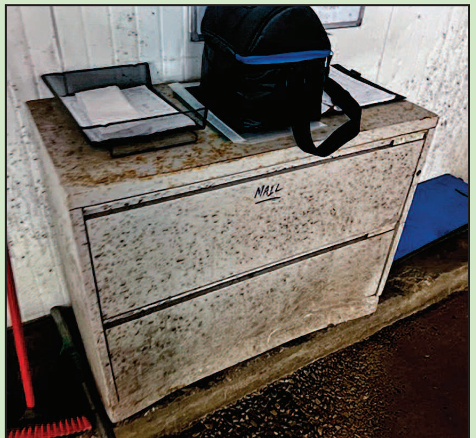
Black mold covers this filing cabinet in the Borden-Select receiving dock of the cold storage area at Franklin Park, Illinois. What a disgusting, dangerous mess.
