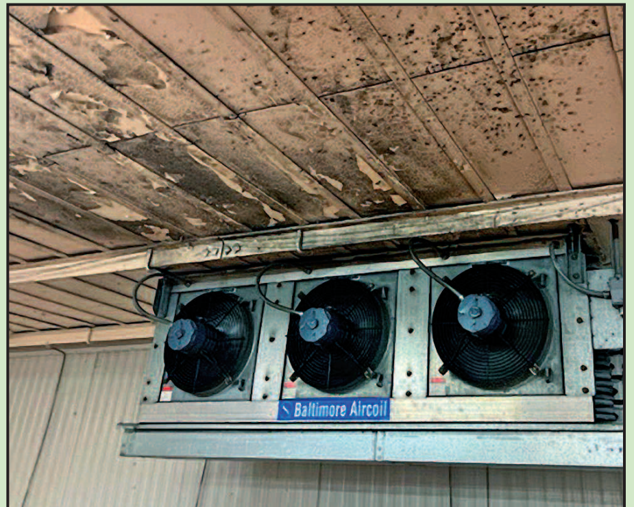
In this same cold storage locker, dirt and black mold are plastered thick, downwind from the ceiling fans. Note the disrepair of the ceiling in this storage area for packaged dairy products. Impossible to clean and sanitize that surface!
